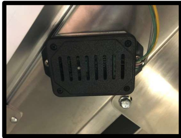
Interior ozone sensor
