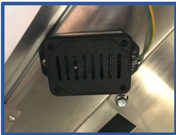
Interior ozone sensor- left
